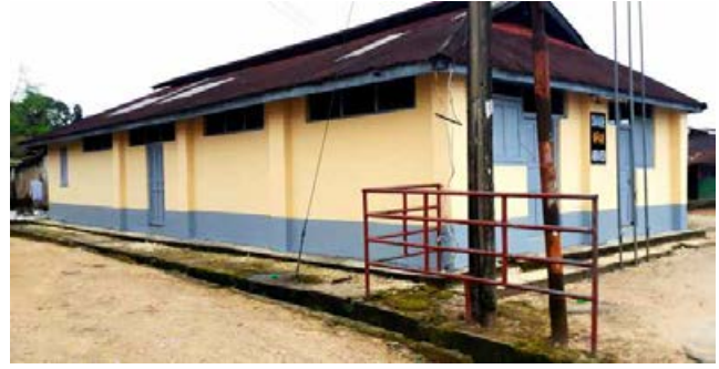
Ekpe Community Hall repainted by the team members at Transcorp Hotels Calabar.
